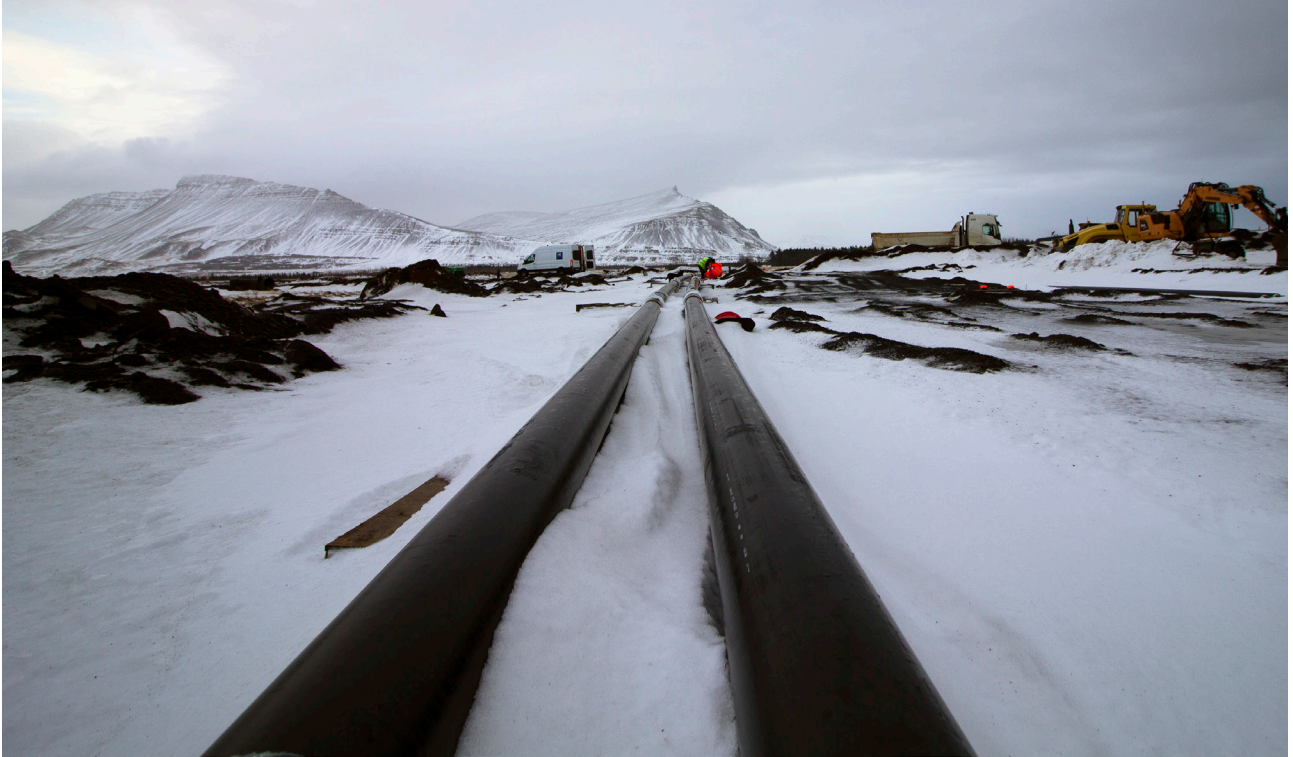
Central heating pipes used in Reykjavík, located in Akranes.
